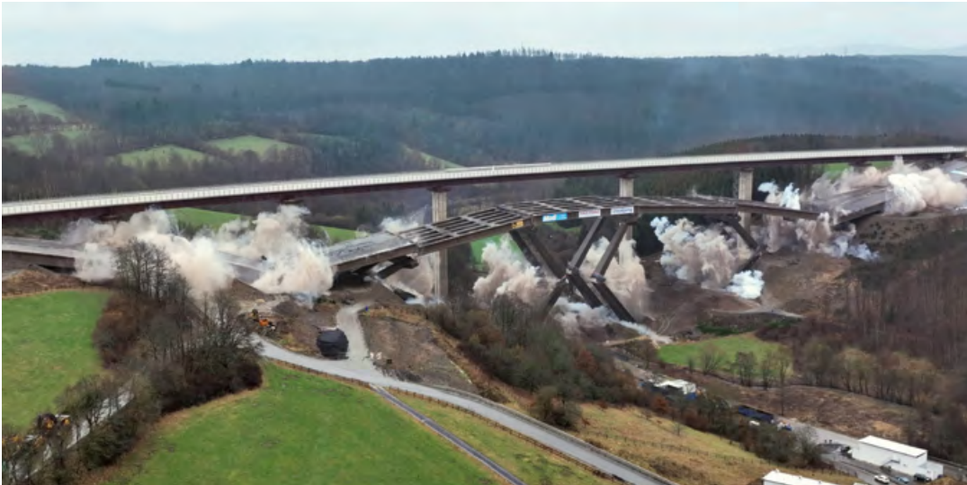
500 meters long and 70 meters high, the Rinsdorf viaduct on the A45 imploded on February 6, just as planned — right down to the centimeter level. Under no circumstances could the demolition be allowed to damage the first part of the new bridge, which stood directly alongside.
